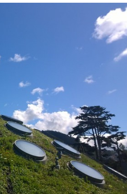
Top: Green roof of the California Academy of Sciences (2014). Image by Ruth Hartnup/Flickr. Licensed under CC BY 2.0 . Original location here .
