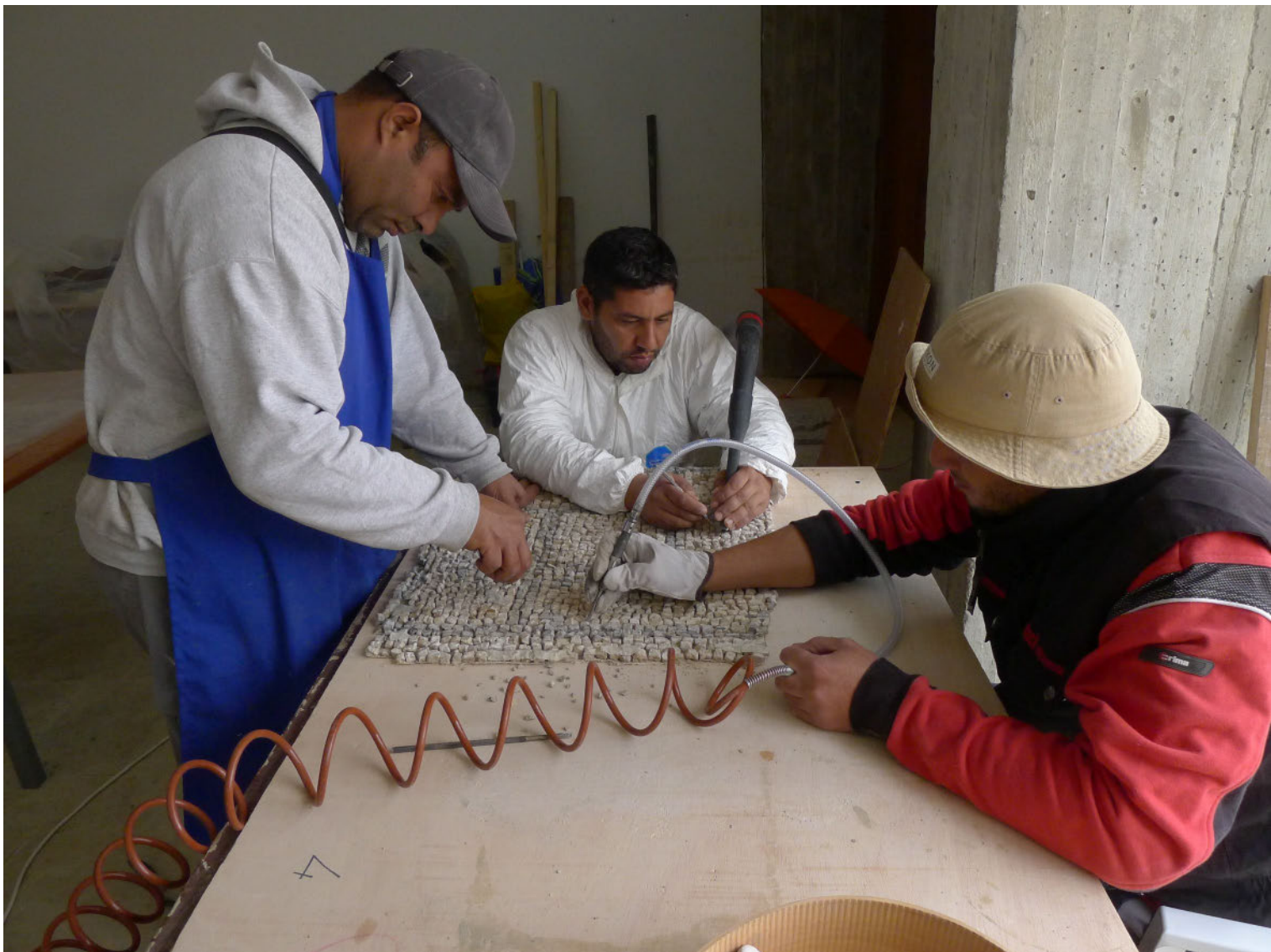
Practical training in mosaic conservation in the Maison de la Chasse, Bulla Regia, Tunisia, a collaboration of the Getty Conservation Institute, Institut National du Patrimoine de Tunisie and World Monuments Fund. (Scott Warren, © 2011 J. Paul Getty Trust)
