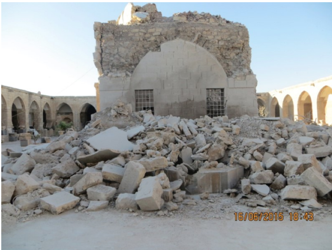
A photograph of the heavily damaged al-Ma'ara Museum taken by local partners (photograph provided by The Day After - Heritage Protection Initiative; June 2015)
