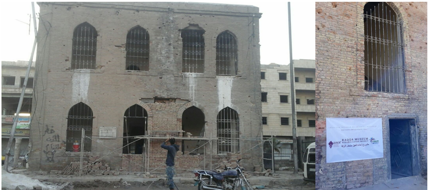
(Left) The heavily damaged Raqqa Museum. Image taken by an ASOR CHI partner. Image courtesy of ASOR CHI. (Right) A photo of the Raqqa Museum with the “Rehabilitation Project” banner. Image courtesy of ASOR CHI
