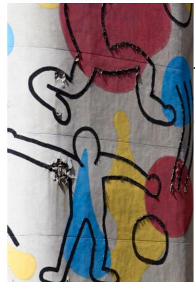
Detail of deterioration on the south side of the mural, 2012.
