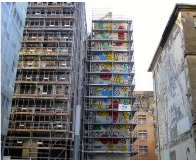
Unwrapped scaffolding reveals cleaned mural before demolition of the surgery centre (left).
